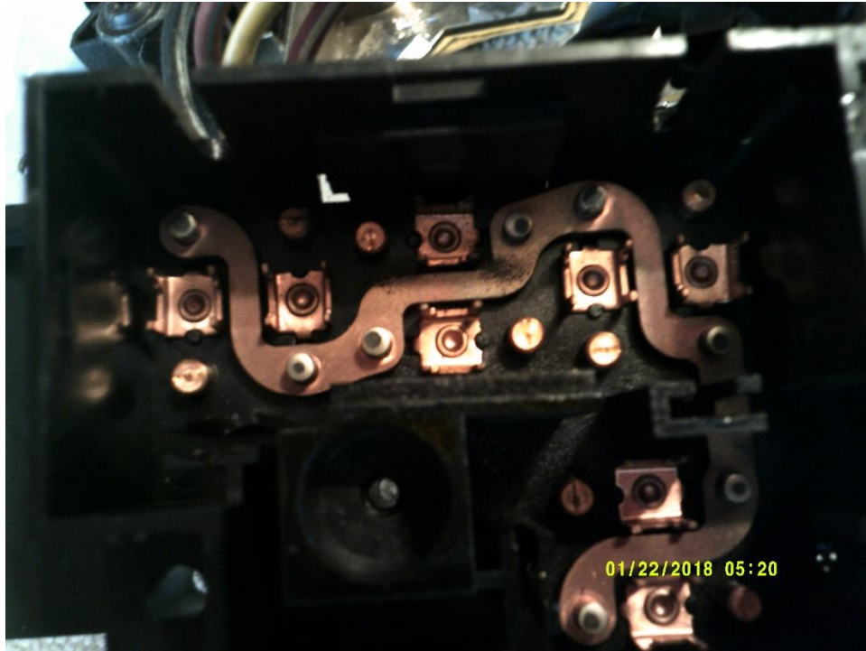
Inside the switch with parts removed. Where stick was used.
